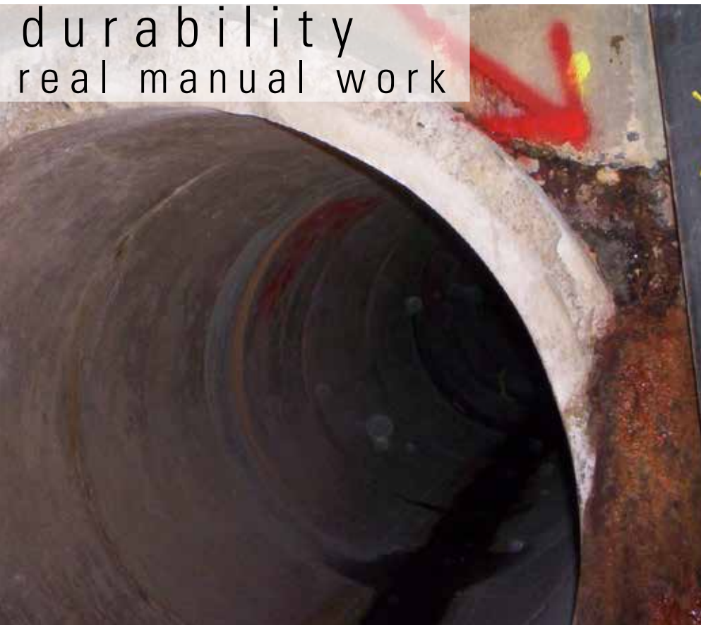
Groundwater ingress at shaft connection
