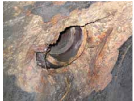
Pipe socket before the rehabilitation
