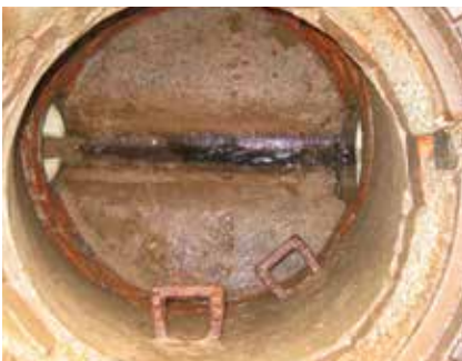
Before the rehabilitation
